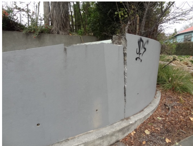
Figure 7. A typically damaged concrete retaining wall
