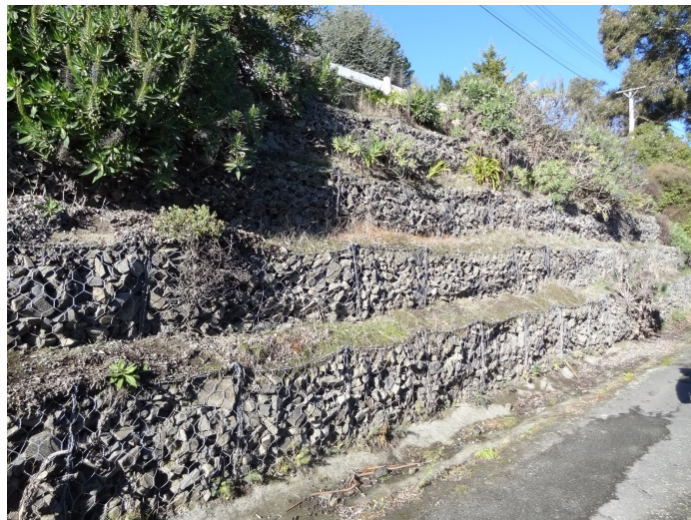
Figure 5. A badly deformed gabion wall
