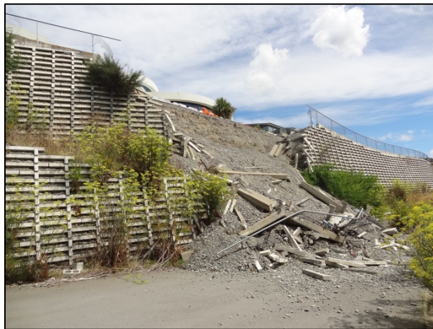
Figure 1. An example of a collapsed crib wall
