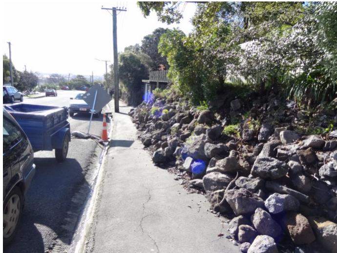
Figure 9. A completely collapsed stone wall
