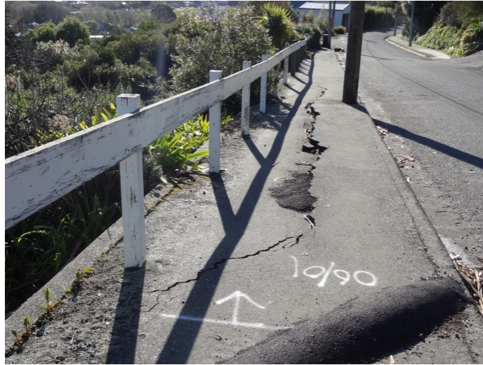
Figure 6. Footpath above a gabion wall showing cracking
